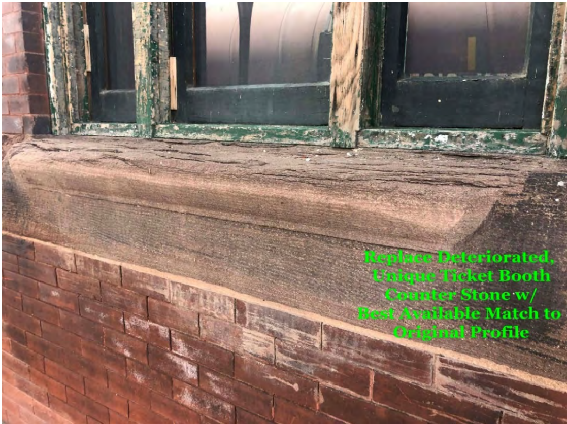
Example of sandstone window sill restoration needed
