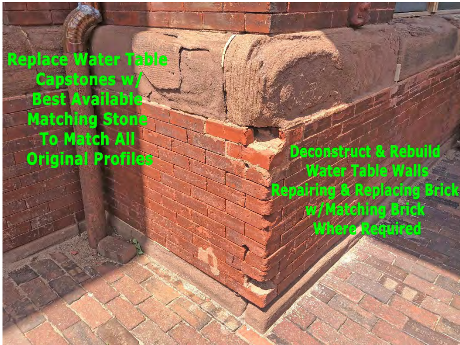
Example of sandstone and brick restoration needed
