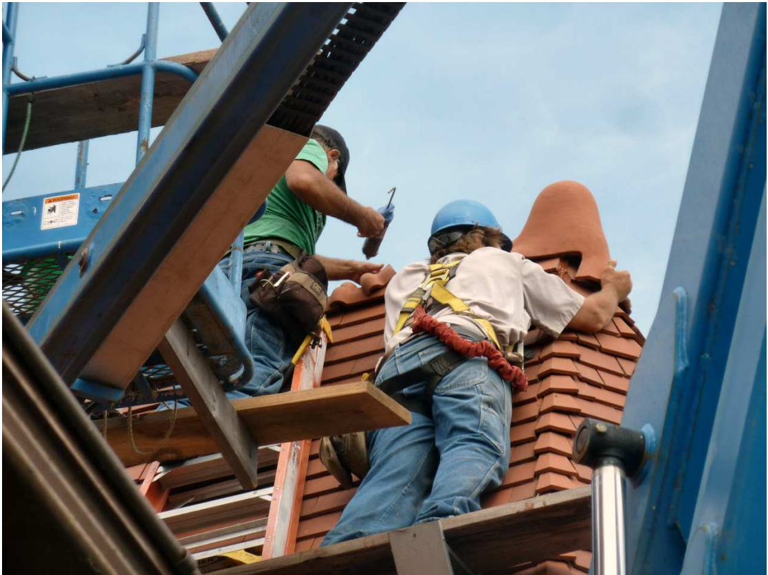
The CCS crew installs the final tiles on October 8, 2018 Photo by Richard C. Leonard
