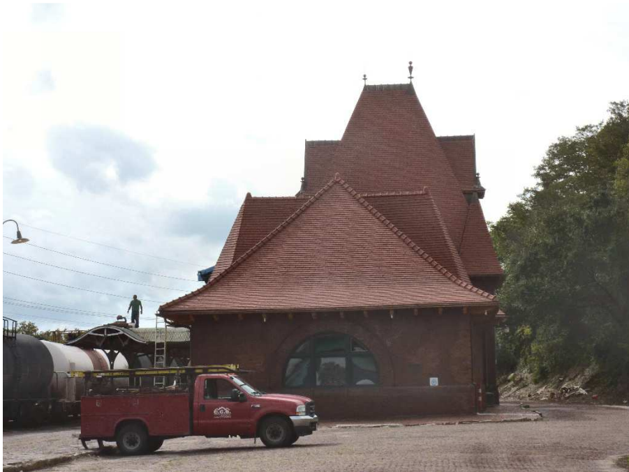
Keokuk Union Depot after completion of the tile installation on October 8, 2018 Photo by Richard C. Leonard
