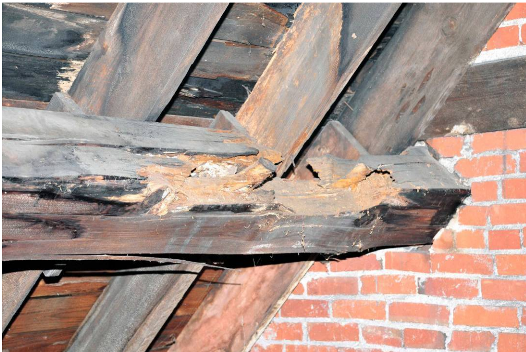
Fig 21. A rotted purlin on the north slope of the downriver roof at the two-story wall.
