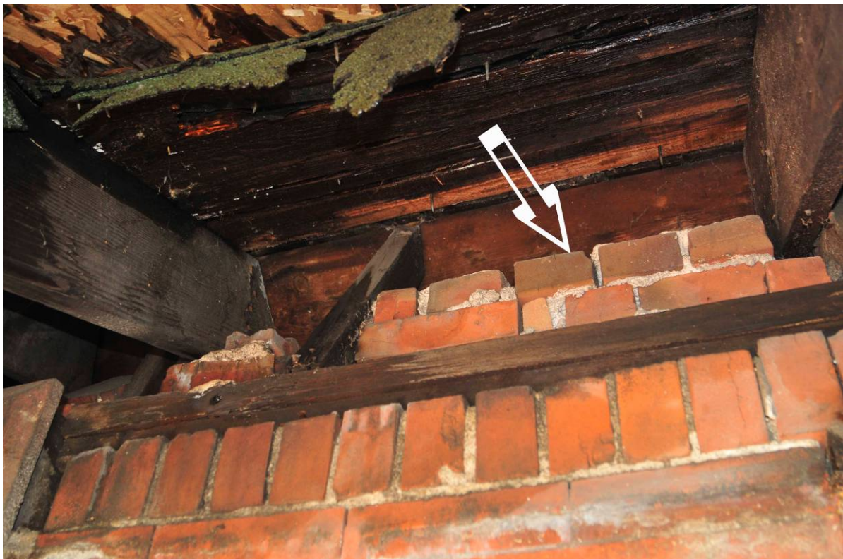
Fig 26. Face bricks atop the wood top-plate can be salvaged for visible repairs below the eaves.
